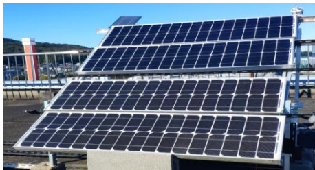
Fig.6 PV array used in the experiment.
