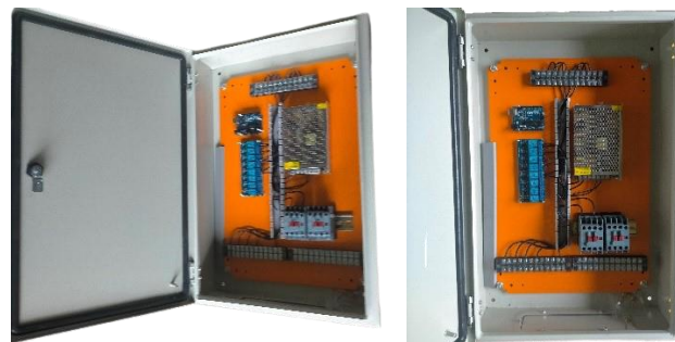
Fig. 2: Controller Circuit Panel Board
